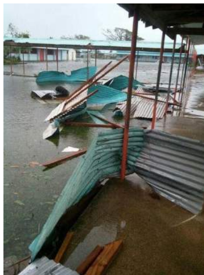
Above: Ekuasi Manu | Damage at Apifo'ou College from Cyclone Gita.
