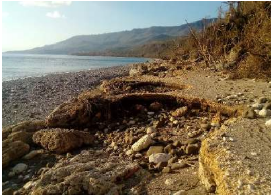
Parts of the road between Melsisi and Lonorore Airport that were damaged by the sea
